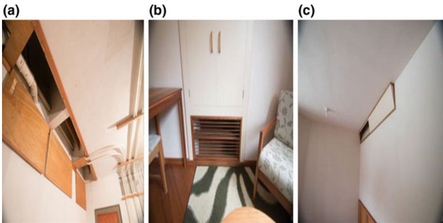
Fig. 6 Ducts for vertical ventilation
